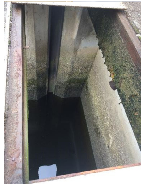
Photo 6 North Gate Slot - Embedded Steel Guide ( 2023-08-22_09h-26m.jpg )
