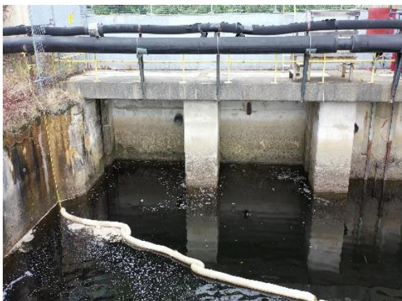
Photo 5 Unit 8 Wingwall, South and North Draft Tube Bays (DJI_0187 - frame at 0m7s.jpg)
